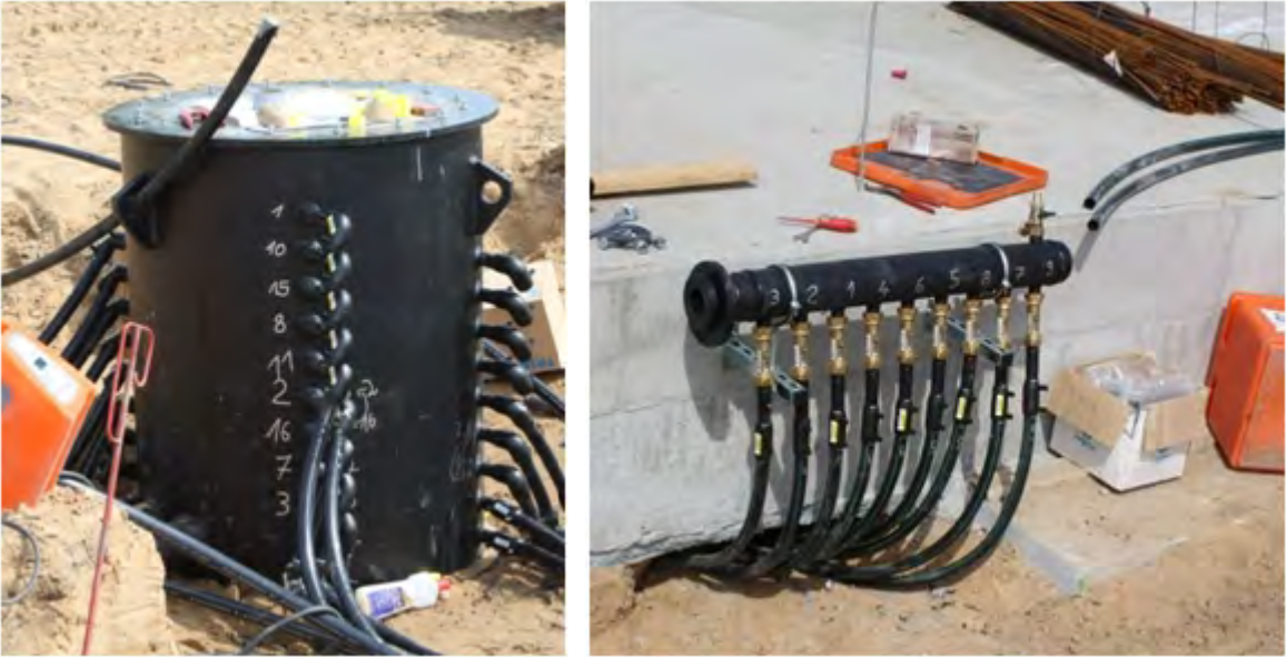
Fig. 95. left: collector/distributor shaft; right: header pipe with 9 individual circuits attached; both images taken in Stade, Germany.
