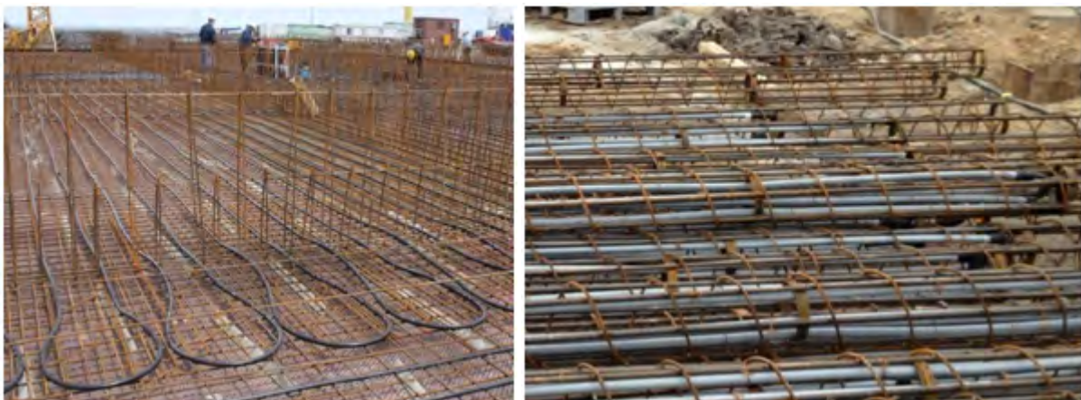
Fig. 93. left: thermal activation of a base plate in the harbour area of Hamburg, Germany, piping material: PE-RC, 25 mm; right: thermally activated foundation piles in Rostock, Germany, piping material: PE-Xa, 25 mm.
