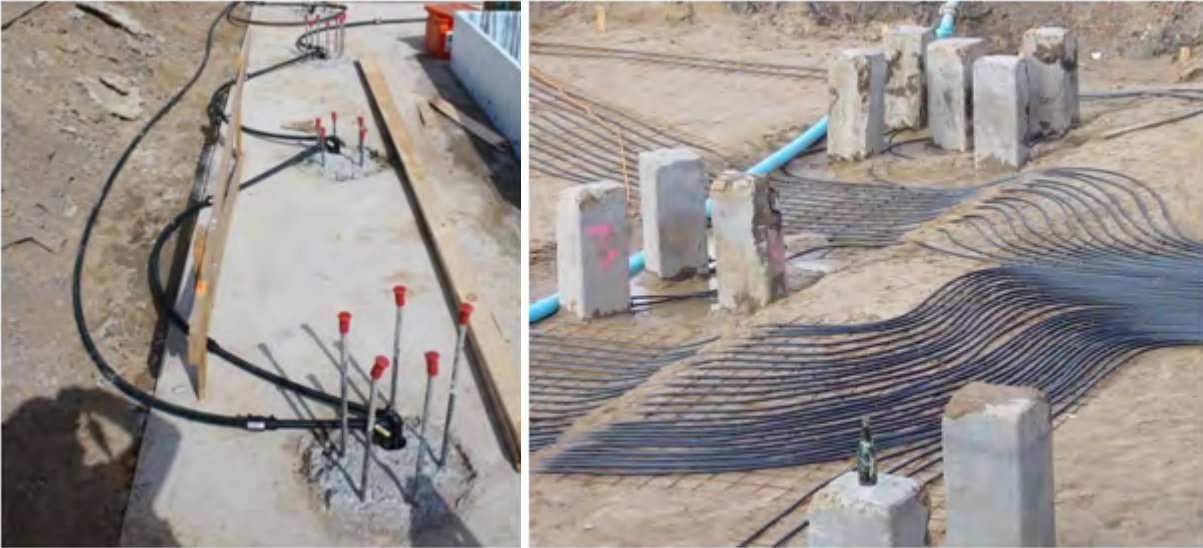
Fig. 94. Two examples for hydraulic connection of energy piles; left: Stade, Germany; right: Rostock, Germany.
