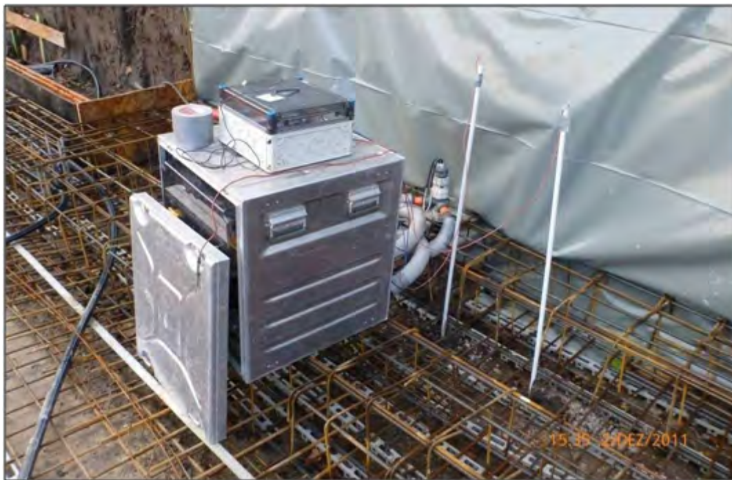
Fig. 19. Setup of the GRT and temperature measurement on the energy pile in Oldenburg. The metal box contains the GRT instrument; temperature sensors are located inside the pile as well as in two distances to it, visible here by the white PVC-pipes pointing out of the ground.
