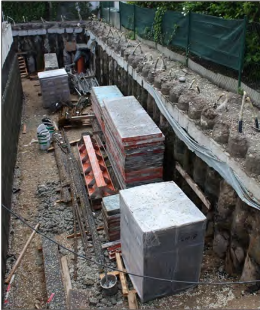
Fig. 15. Construction of a thermally activated bore pile wall in Rostock, Germany. every second segment of the wall is thermally activated, as can be seen by the PE-pipes pointing out of the individual segments.
