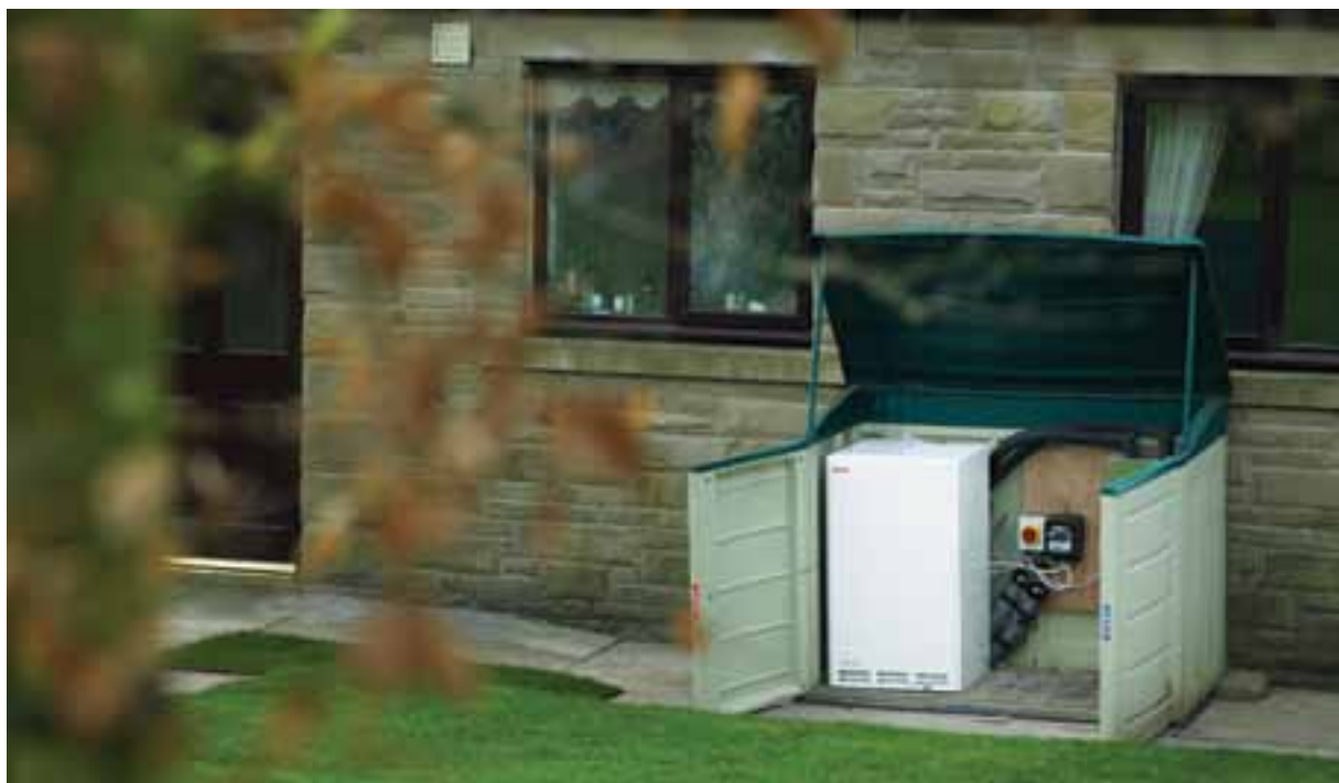
The above-surface part of a ground source heat pump
