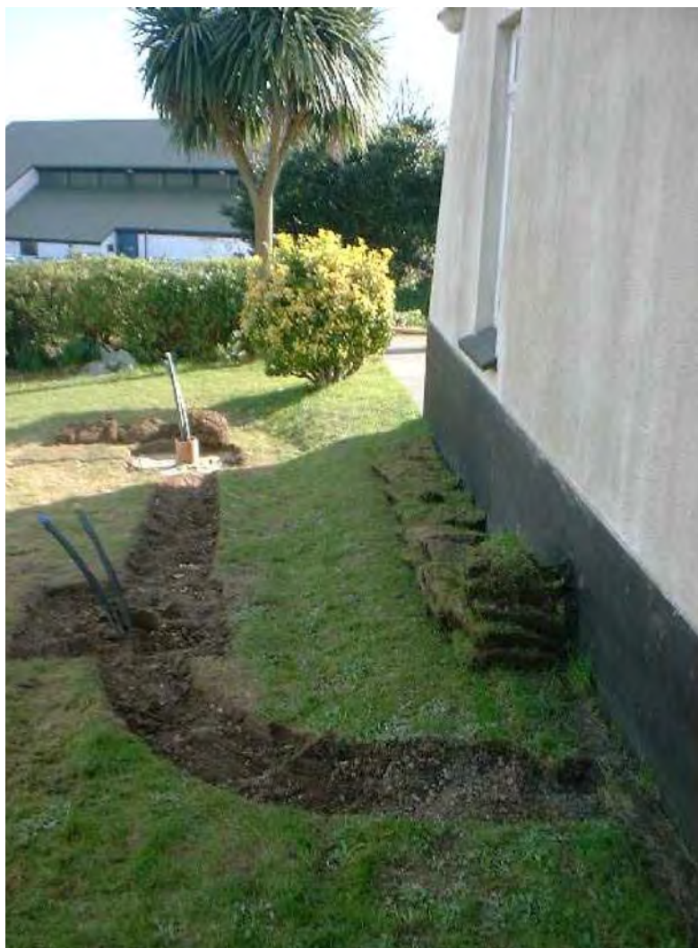
Figure 9 The heating needs of this house are supplied by a vertical collector GSHP system © Robin Curtis
